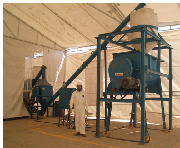
Fig. 1. Picture of the pilot plant implemented to treat COPR.
